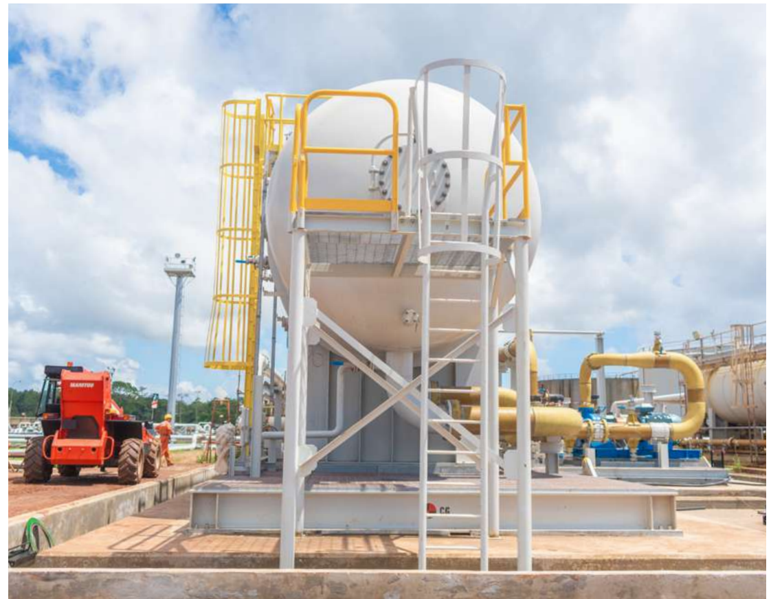
ISF-3 unit at Gamba Terminal in November 2023.
