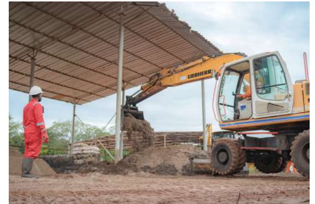
2 Nutrients are added and aerated to improve efficiency of treatment process.
