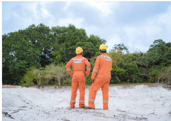
4 Once treated to within internationally compliant levels, soil is used to backfill excavated land and is covered with an ecolayer to encourage regrowth.
